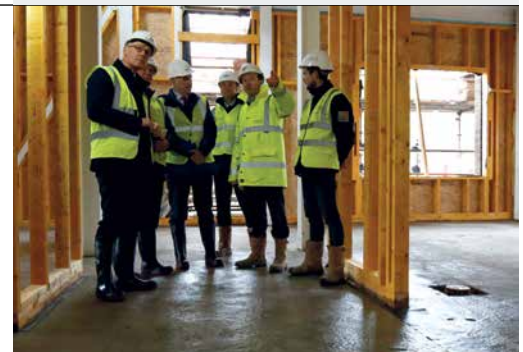
The Deputy First Minister with Professor Alex McMahon (NHS Lothian), Paul McGirk (Hub South East), Andrew Milne (NHS Lothian), David Wilson (Morrison Construction) and trainee William Johnstone on site at the new brain injuries unit
