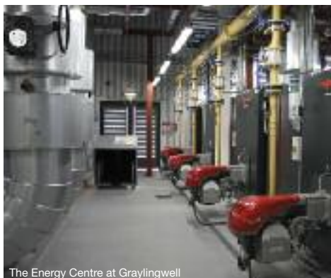
The Energy Centre at Graylingwell
