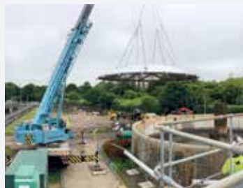
● AMP6 - Yorkshire Water, Scottish Water and Southern Water
